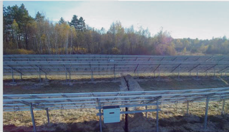
Ukraine 15MW Solar Plant
