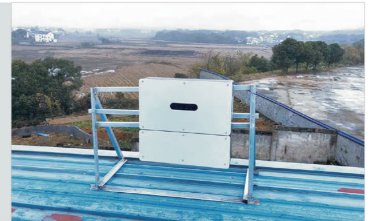
Roof-top PV Project in Hunan China
