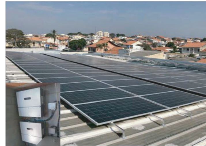
Brazil 500kW Rooftop Project
